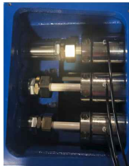
(Figure 5.1.13) Plunger installation
